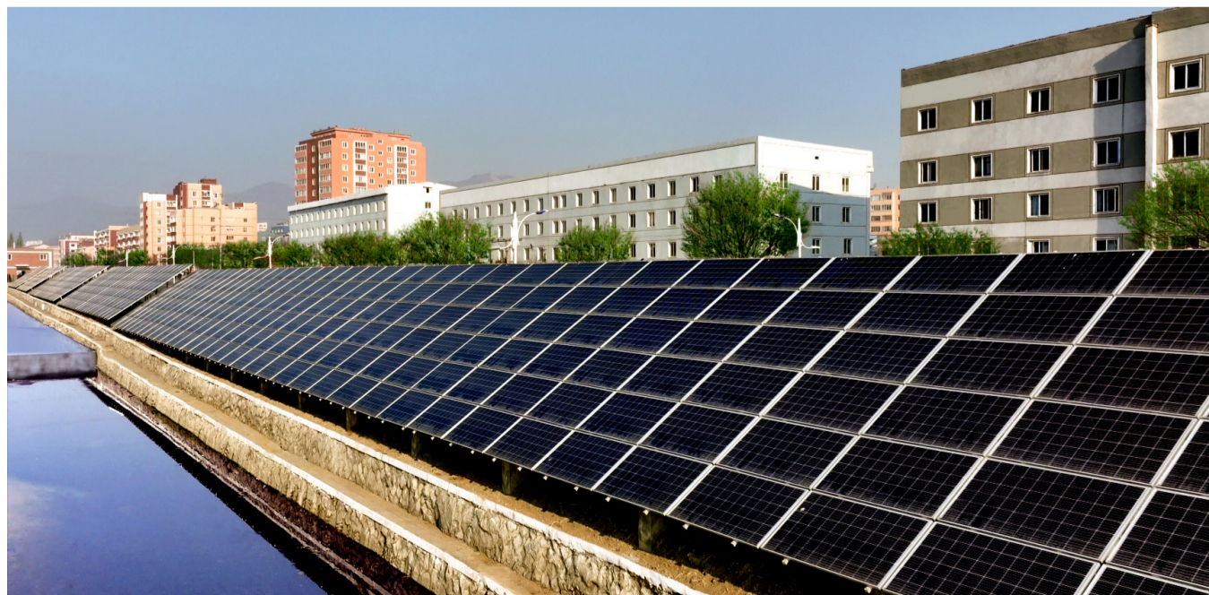
Solar panels produced by the Jinung PV Module Factory of the Jinung Trading Company are installed in the city of Phyongsong, South Phyongan Province.
