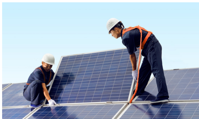
Employees of the Jinung PV Module Factory of the Jinung Trading Company install solar panels. RYU KWANG HYOK/THE PYONGYANG TIMES
