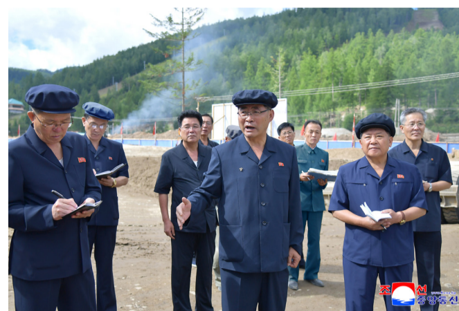
Premier Pak Thae Song (middle) inspects the construction site of the Samjiyon Tourist Resort.
